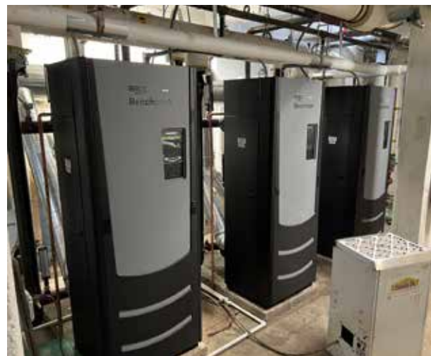
In 2022, new boilers were purchased and installed. Thanks to all who supported this critical need in building maintenance.
